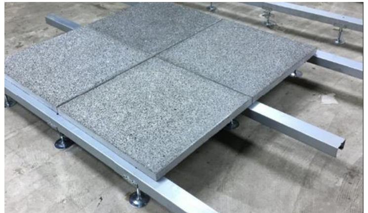
Hot-dipped galvanized steel base beams, and pedestals
